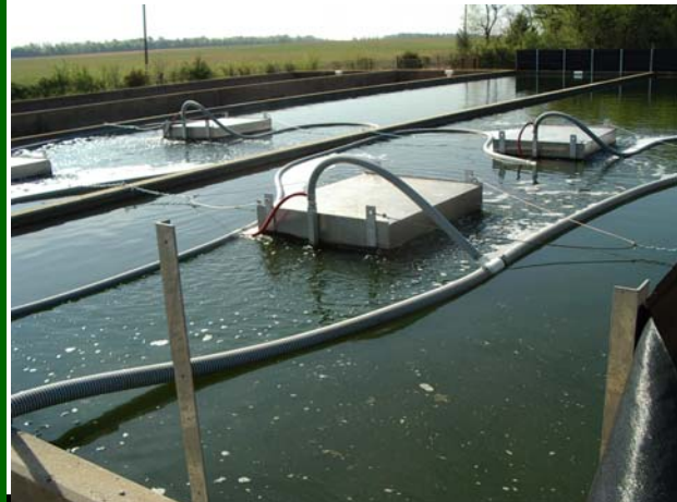
Four new Bio 2 Bloc units were installed in this “recycled” sand filter to improve the removal of ammonia, BOD, and TSS.
